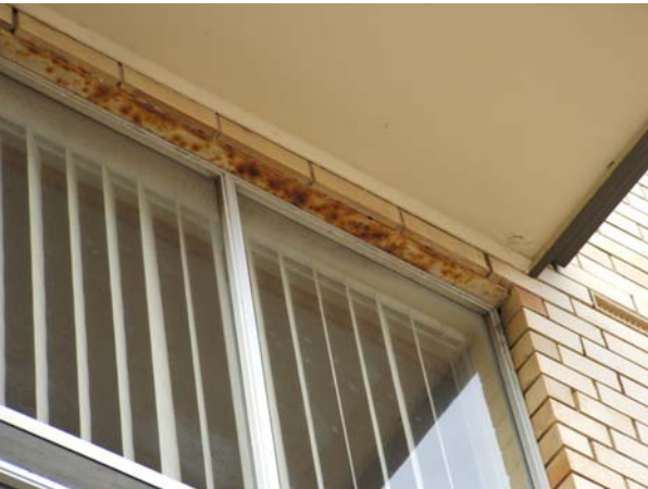
View of window lintel - all show signs of extensive rusting.
