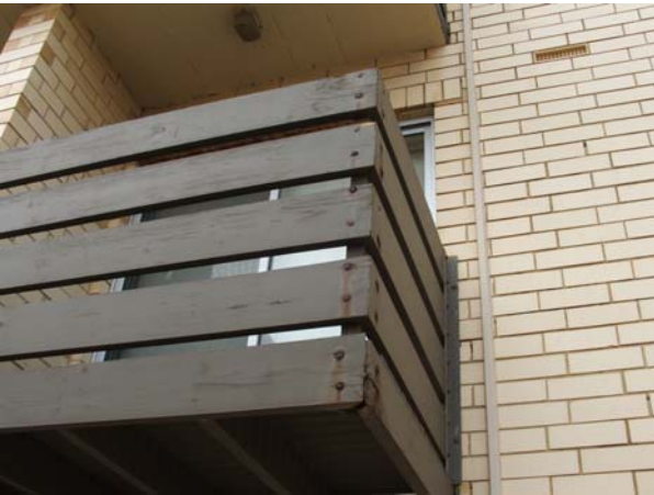
Rusting of steel bolts and some rot evident on this balcony.
